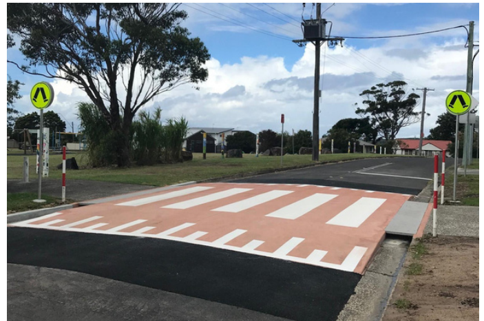
Recently installed School Zone Wombat Crossing at Warilla North Public School (Oldfield Street)
