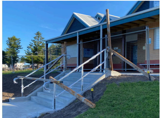
New stairs and paths are being installed at Beverley Whitfield Pool to improve access at the facility.
