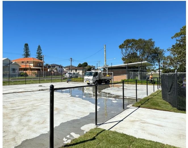
The new multipurpose court at Dawes Park in Barrack Point is currently under construction. Once completed, this public court will be marked for basketball, futsal, and pickleball.
