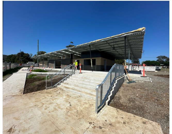
The new amenities and clubhouse building at Albion Oval, Albion Park Rail, is nearing completion. We anticipate its opening in early 2024.
