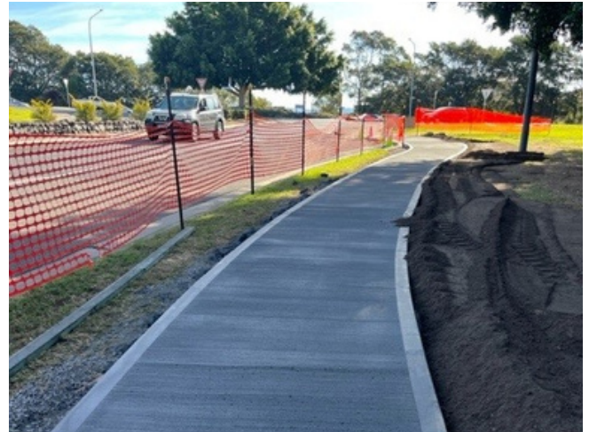
Construction is underway to establish a footpath that will connect the current shared-use paths along Shellharbour Road and Cove Boulevard, Shell Cove
