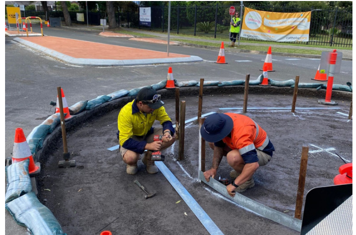
Roundabout construction at the intersection of College Avenue and Glider Avenue, Blackbutt
