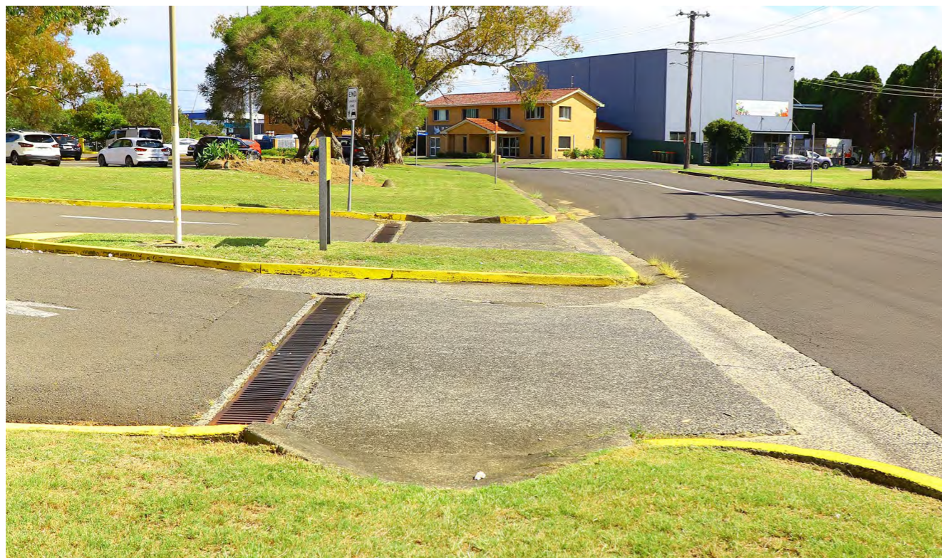
Figure 6.39: Missing footpaths and pram ramps across the car park access to the Warilla Grove Shopping Centre
