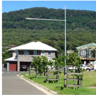
STREET LIGHTING: EDEN POLE
