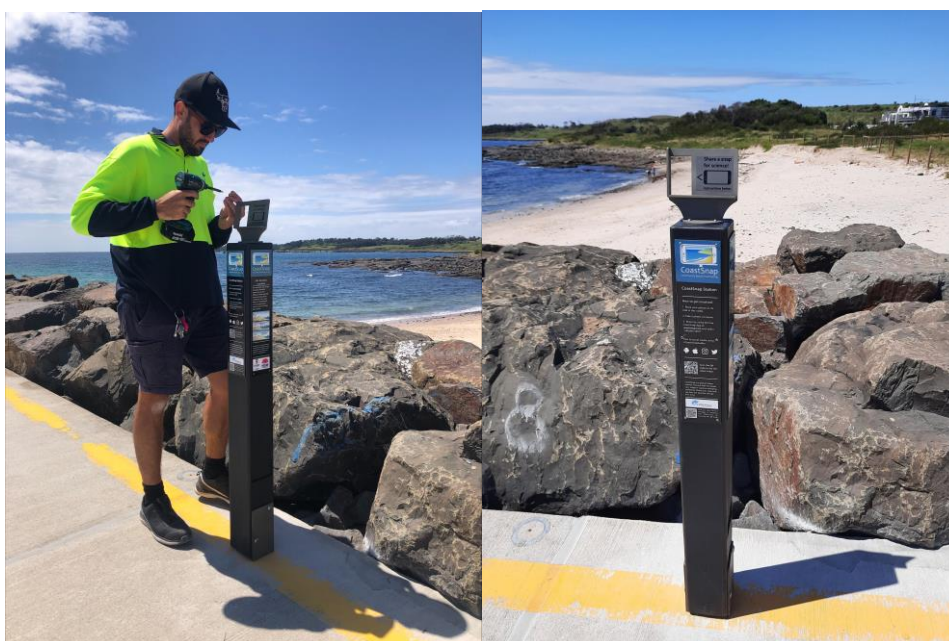
Figure 3: Installation of the CoastSnap infrastructure to monitor Gadhu Beach (installed on Shell Cove Harbour southern break wall).
