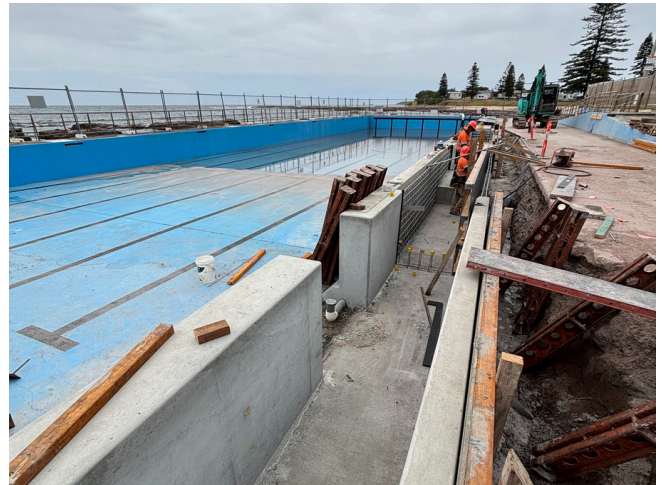
Construction of a new accessible ramp is now underway at Beverley Whitfield Pool, Shellharbour.
